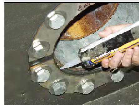
Figure 14. Caulk Exposed Galvanized Steel
