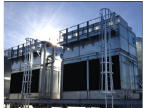
Fluid Cooler / Closed Circuit Cooling Tower
