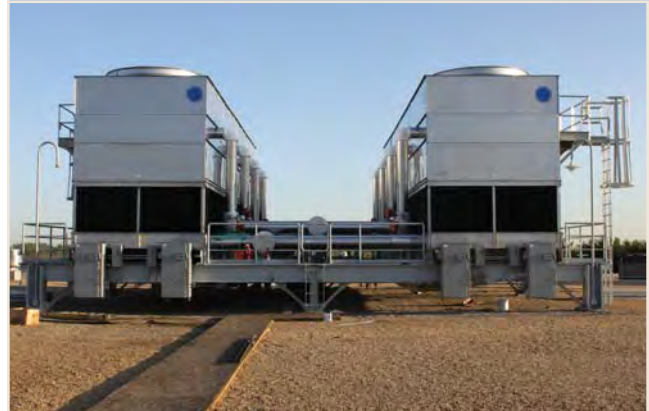
PHOTO 2 Multi-cell counterflow open circuit cooling tower installation.
