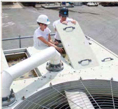
PHOTO 3 Regular cooling tower maintenance pays off.
