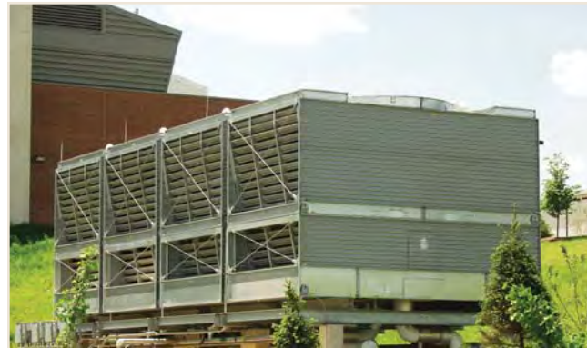
PHOTO 1 Four cell crossflow open circuit cooling tower.
