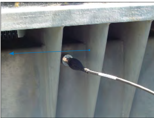
Figure 11a. Accelerometer Location - Gear Drive
