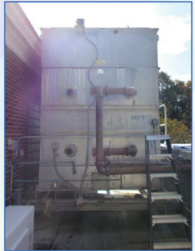
Less than one foot clearance between the original unit and parapet wall made maintenance extremely difficult.
