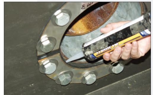
Figure 13. Caulk Exposed Galvanized Steel
