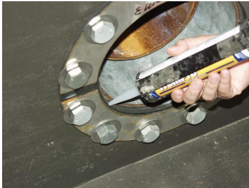
Figure 75. Caulk Exposed Galvanized Steel
