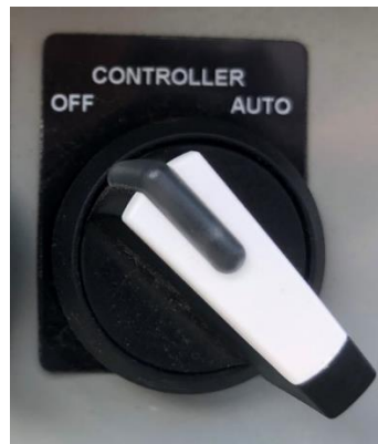
Figure 28. Controller Switch (Local Enable)
