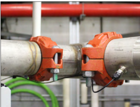
Figure 28. Leaving Process Fluid Temperature Sensor
