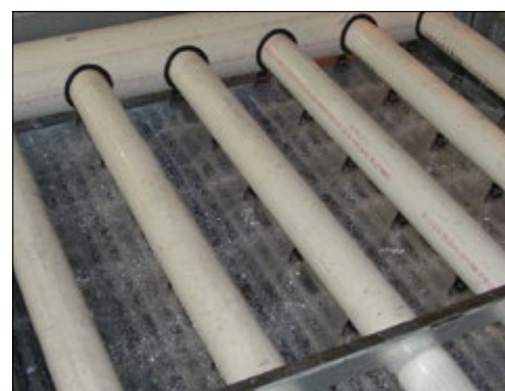
Pressurized Spray Distribution
