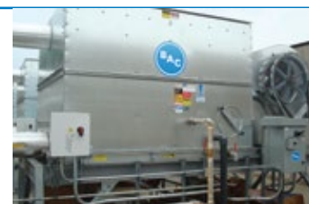
VTL Cooling Tower
