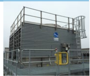
Series 3000 Cooling Tower
