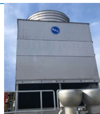
PT2 Cooling Tower
