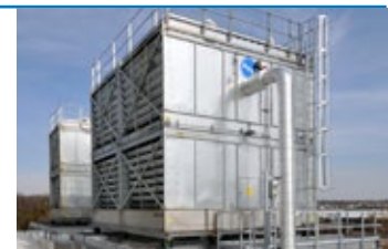
Series 3000 Cooling Tower
