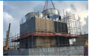
Series 3000 Cooling Tower
