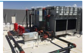
FXV Cooling Towers
