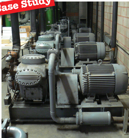
These Carrier open-drive reciprocating compressors were part of the Food 4 Less supermarket's refrigeration system that was converted from R-22 to R-407F by RSI of West Sacramento. (Photo by Ted Rieger)
