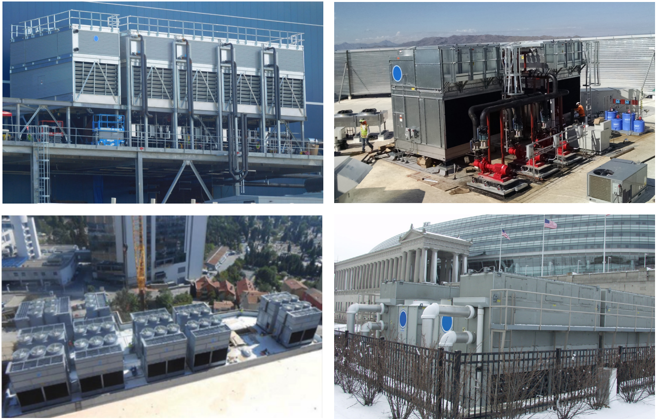
Figure 16 Closed Circuit Cooling Tower Installations
