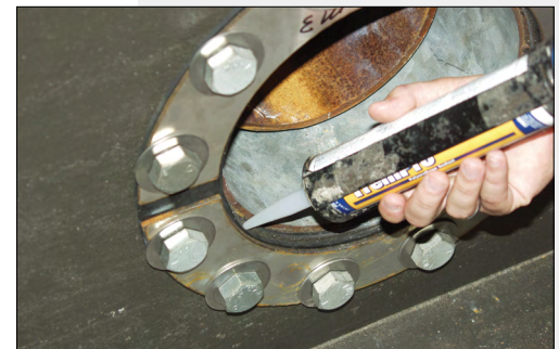
Figure 13. Caulk Exposed Galvanized Steel
