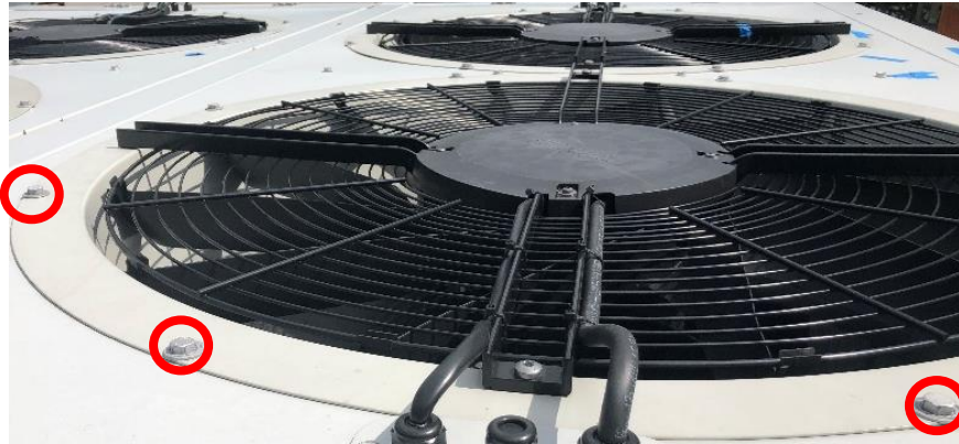
Figure 28. Fan Deck Fasteners
