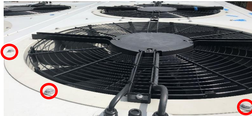
Figure 22. Fan Deck Fasteners
