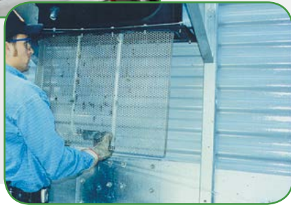
Inlet strainer inspection for Series 3000
